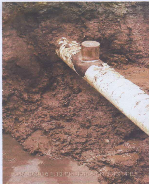
Fig 3: Leak point after repairs
